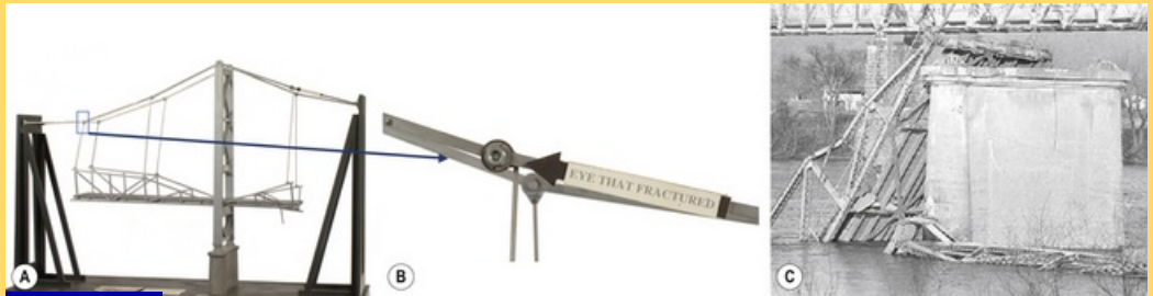
Fig. 4.17 (A) The Silver Bridge showing the eye bar where a defect occurred around the pin (B). This eventually led to a stress corrosion fracture and the collapse of the bridge (C).
